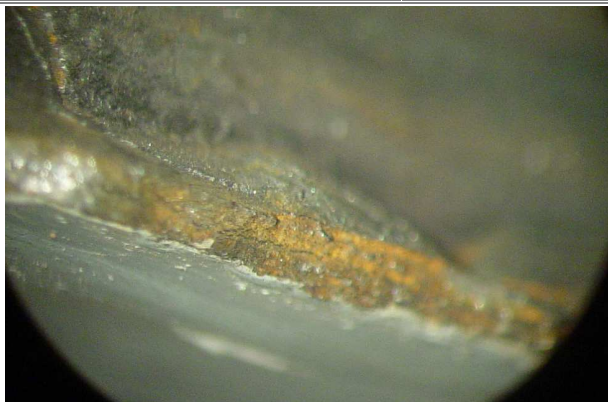
Photo 25: Fracture surface showing corrosion damages, cabin truss (stereo)
