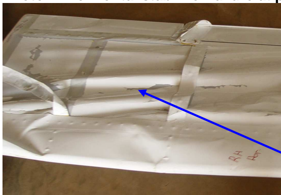
Photo 5: Horizontal stabilizer showing extensive buckling, blue arrow (digital)
