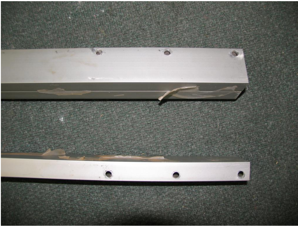
Figure 7. The mast attachment bracket holes which present evidence of elongation
