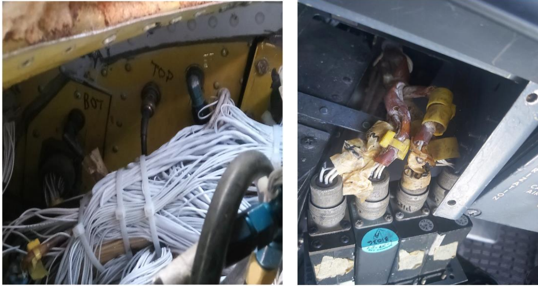
Figures 6 & 7: New wires on the left, and old corroded wires on the right post-accident.
