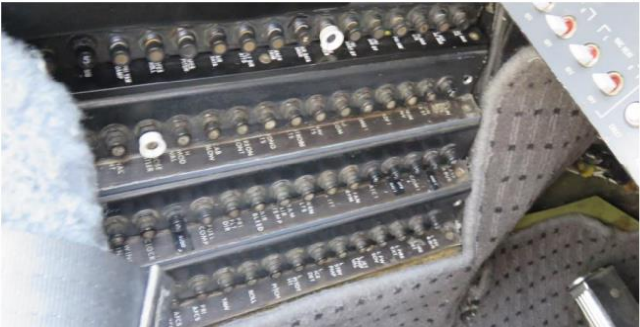
Figure 12: All circuit breakers were in closed position after the accident.
