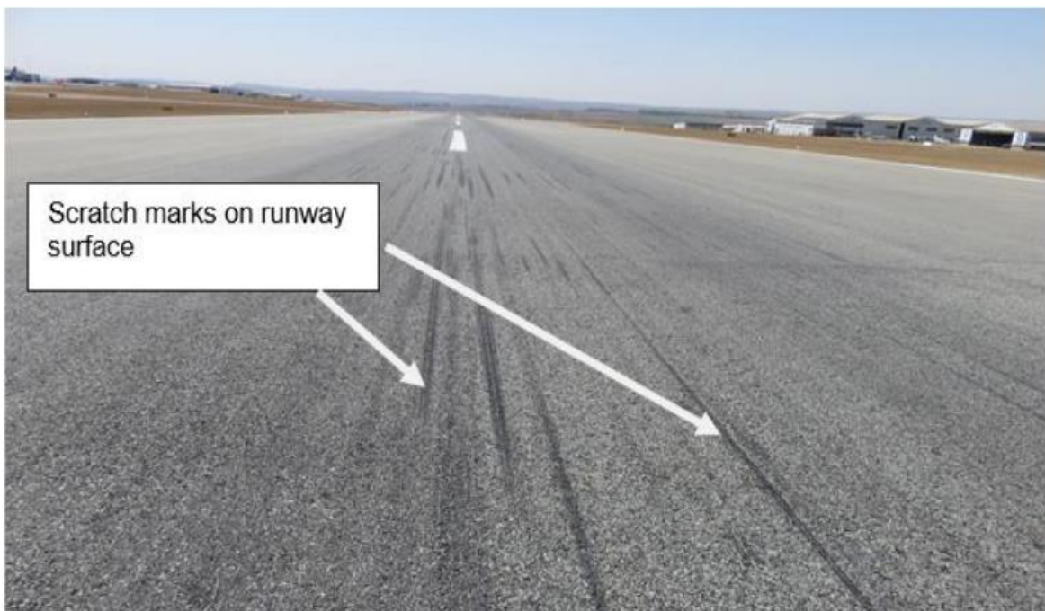
Figure 4: Scratch marks on the runway surface at FALA.
