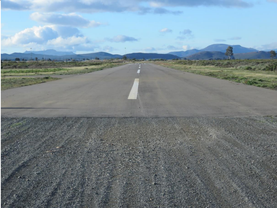
Figure 16: End of the gravel runway surface and the beginning of the last section of the asphalt surface.
