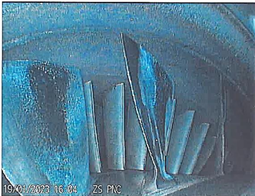
Figure 10: First stage rotor and the stator inlet blades. (Source: AMO)
