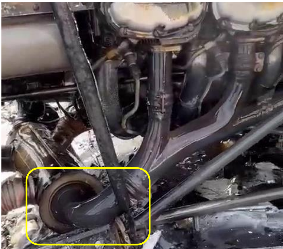
Figure 3: A still picture taken from a video footage of the exhaust system whilst the fire was being doused.
