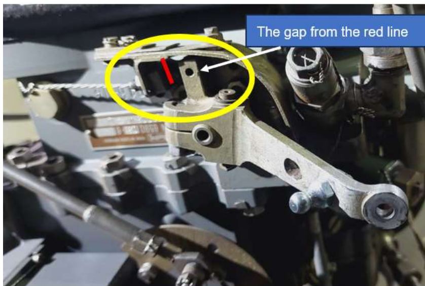
Figure 5: The condition lever which is not at the gate (with a gap).
