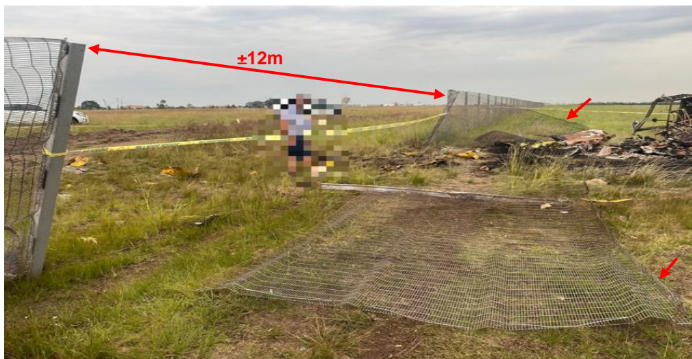
Figure 4: The knocked down perimeter fence on the northern side of the airfield.
