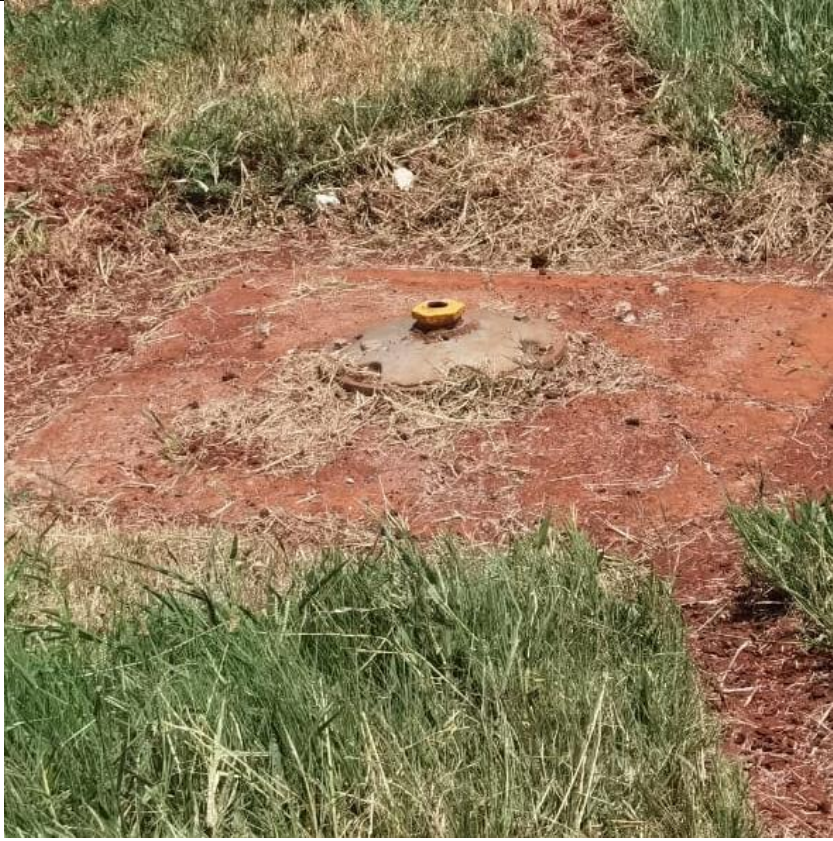
Figure 2: The severed runway light. (Source: ARFF)
