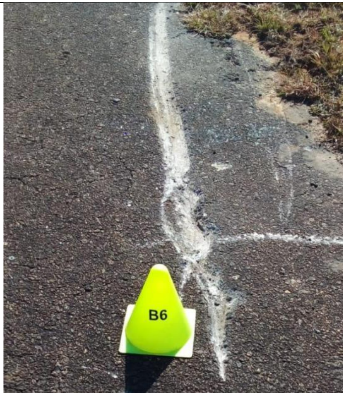
Figure 2: Skid marks on Runway 35. (Source: Operator)
