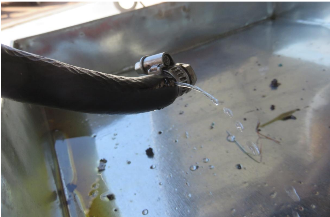
Figure 9: The burst hose was closed at one end; it was filled with water, and pressure was applied by blowing on the other end to identify the area where it had burst.
