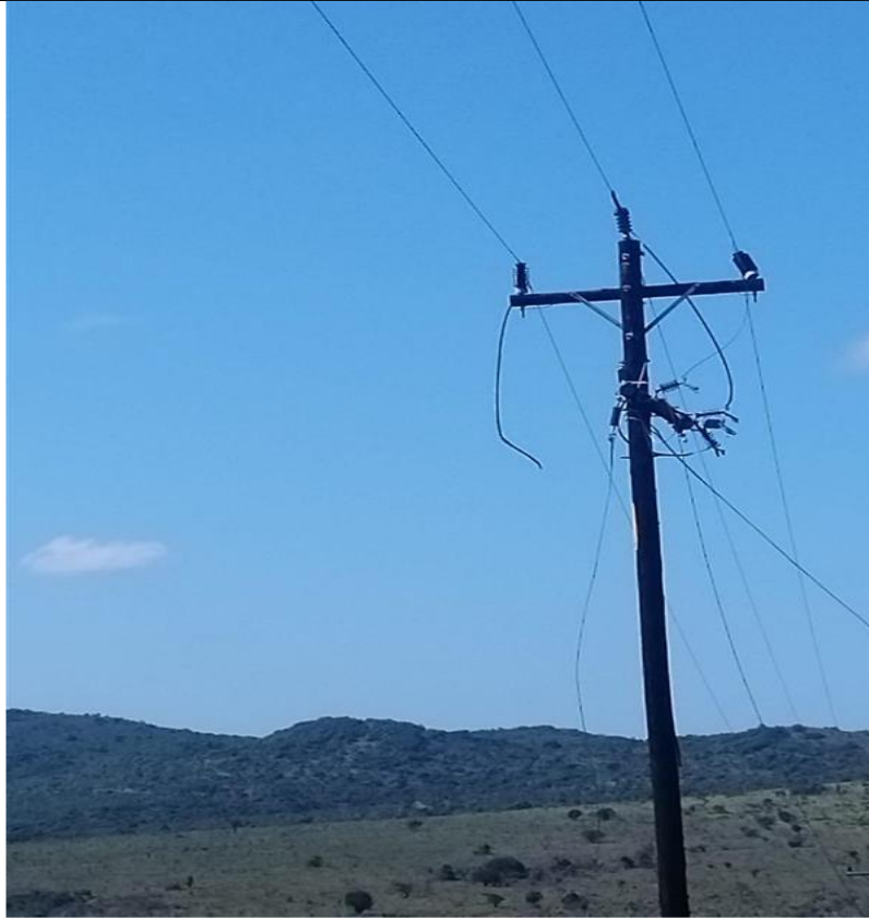
Figure 3: The severed powerlines.
