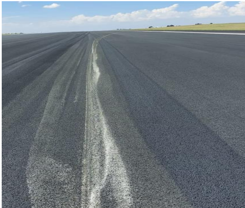
Figure 6: Runway scar mark left by the wing tip as it contacted the runway surface.
