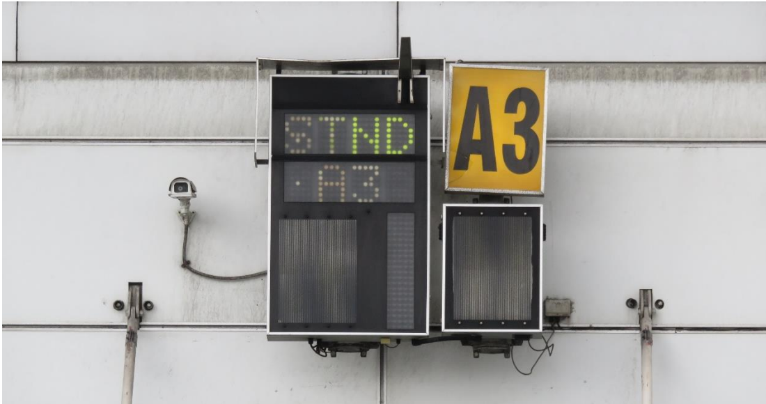
Figure 13: Close-up view of the display unit at parking bay A3.
