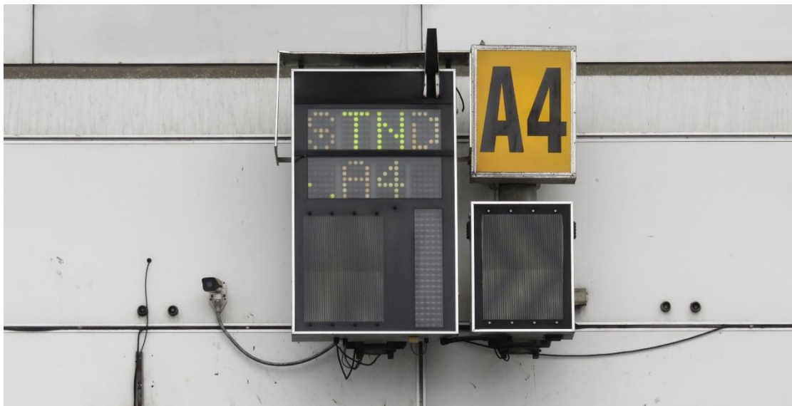
Figure 12: Close-up view of the display unit at parking bay A4.
