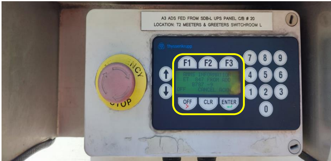
Figure 16: A view of the ADS panel at parking bay A3. (Source: Aerodrome Licence Holder)
