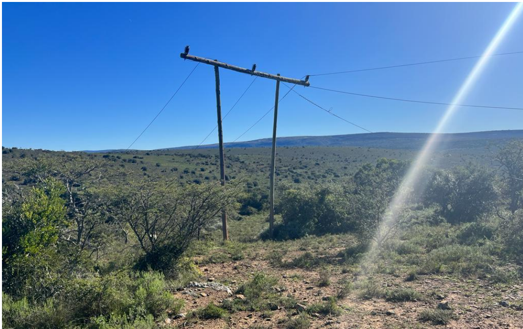
Figure 3: A pylon with all three power lines severed during impact. (Source: Pilot)
