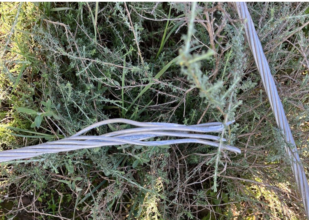
Figure 5: Cables that were severed. (Source: Pilot)
