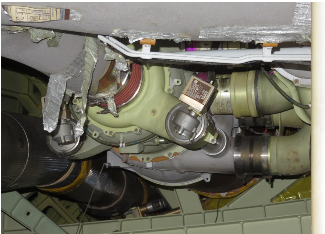
Figure 5: A close-up view of the ACM before removal from the aircraft.
