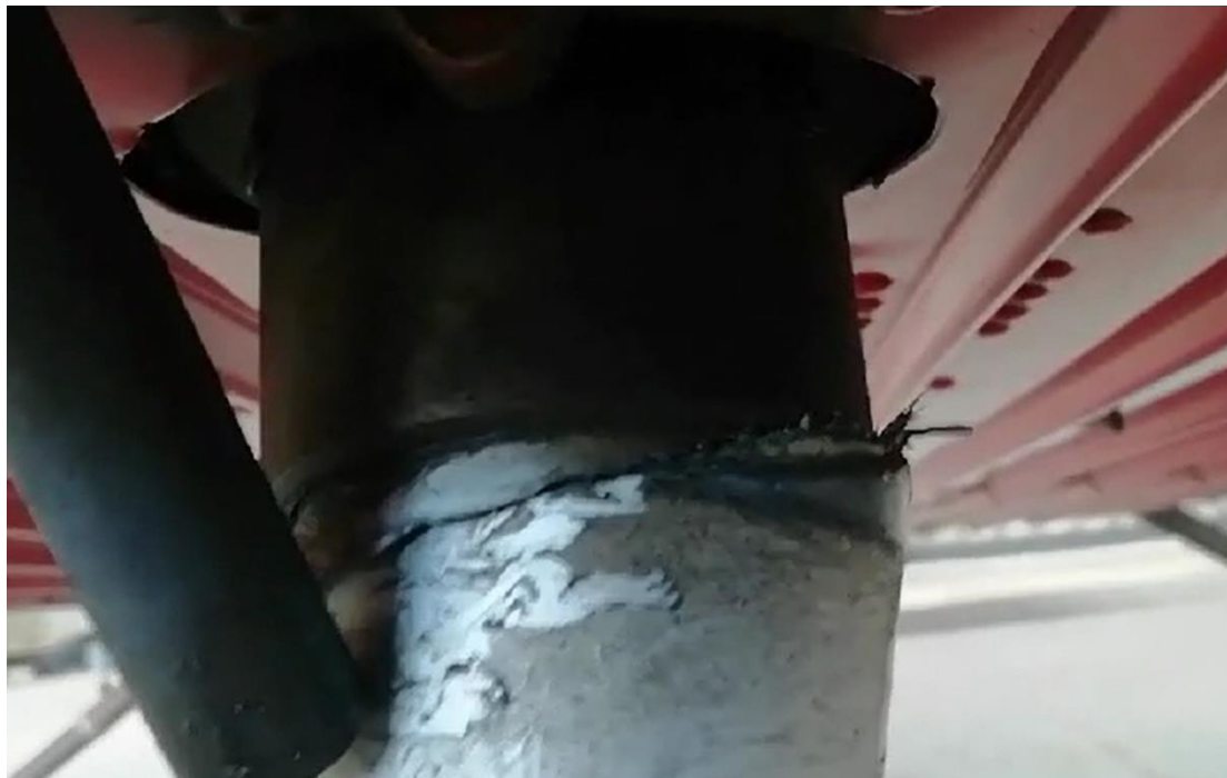
Figure 2: The close-up view of the damaged nose wheel strut. The black pipe is the fuel vent pipe. (Source: Operator)
