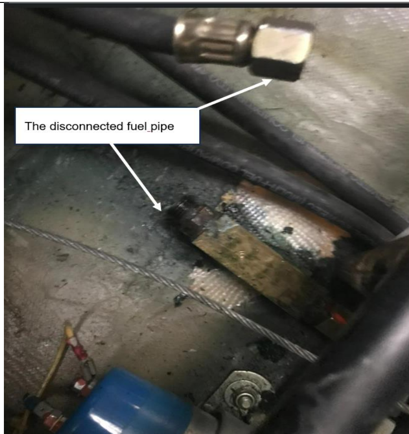
Figure 3: The disconnected flexible fuel pipe. (Source: Engineers)
