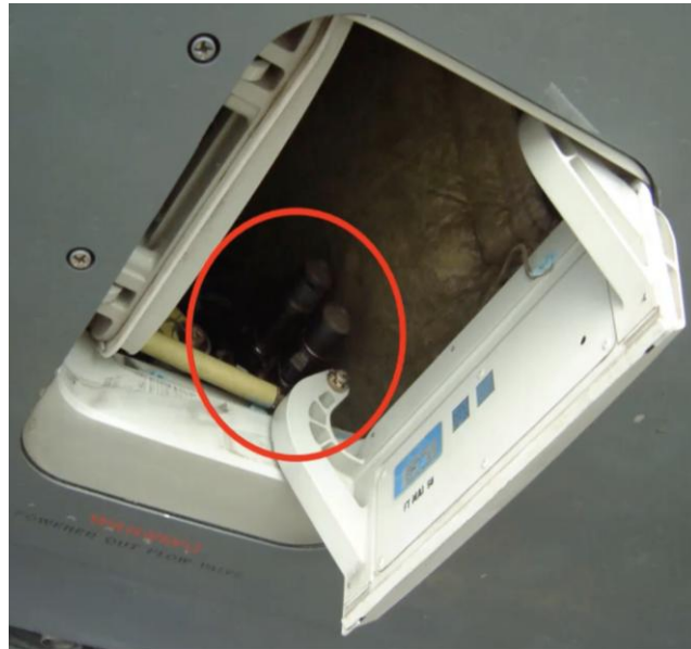
Figure 6: The outflow valve.
