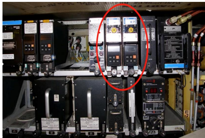
Figure 7: The CPCs as installed in the aircraft electrical and electronics bay.
