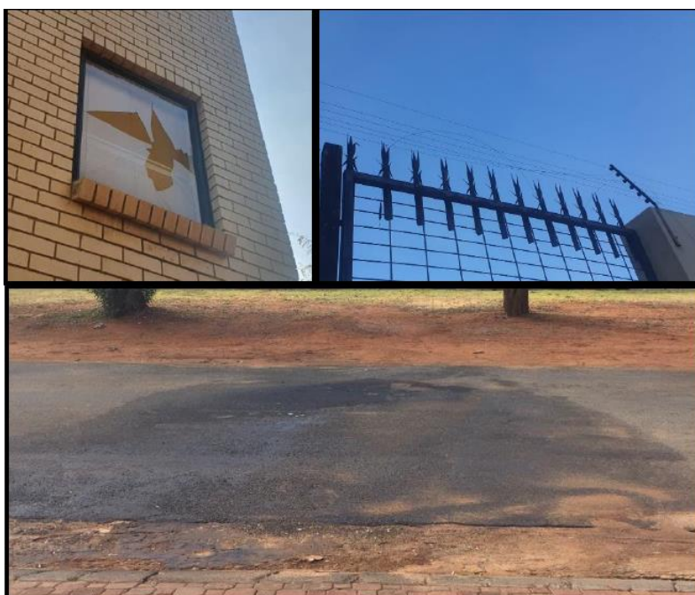
Figure 4: A broken window, severed electric fence and the burnt tarred road surface caused during the accident sequence.
