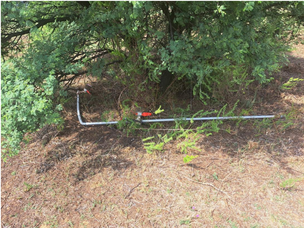
Figure 6: The broken spray system.
