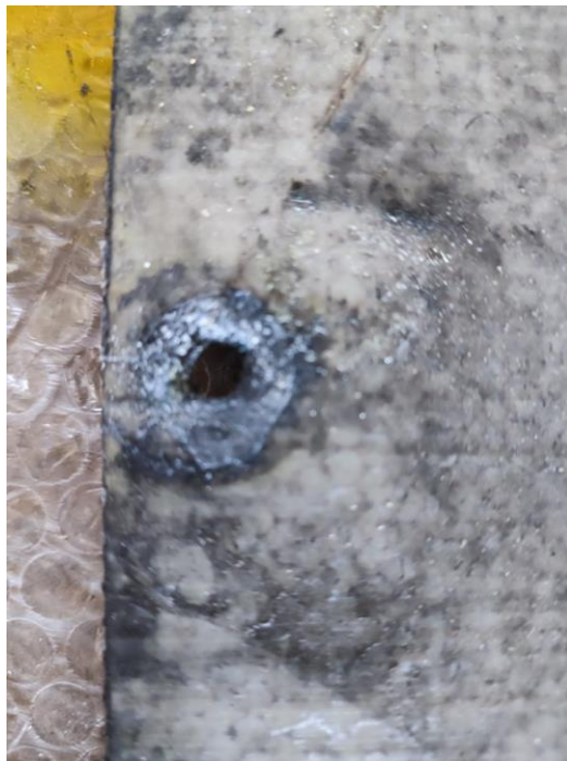
Figure 4. Close-up view of parts of the corroded floor board.
