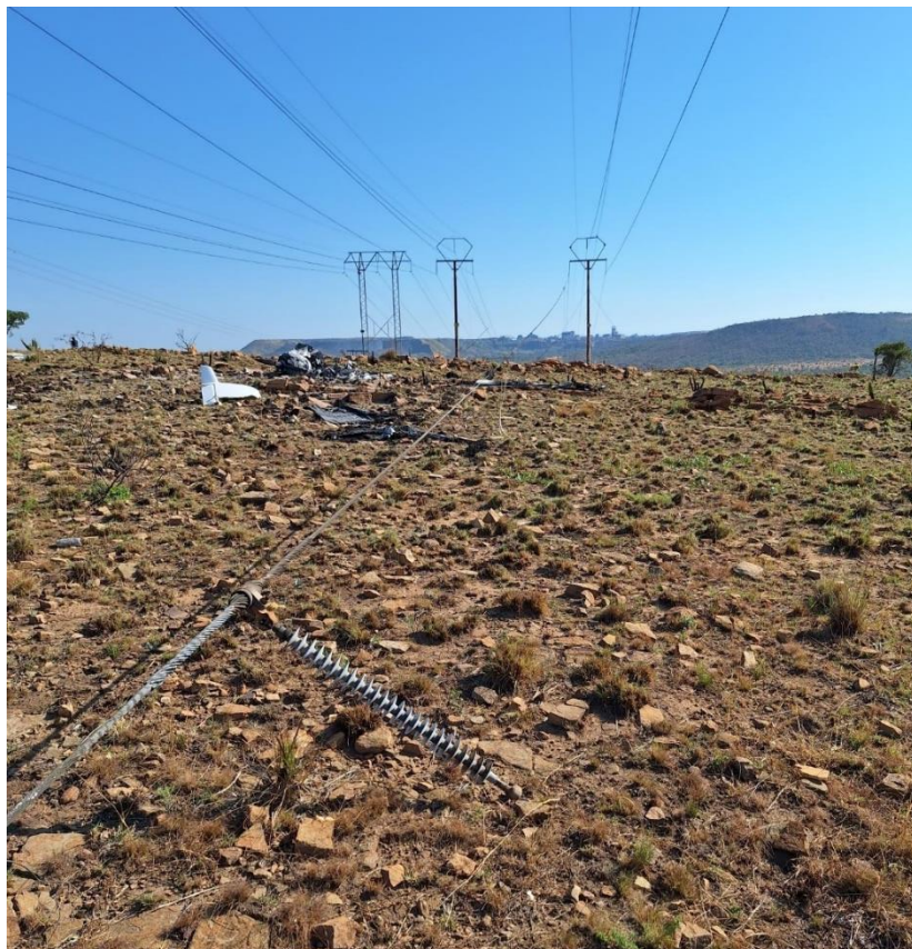
Figure 4: One of the high-tension cables that snapped from the pylon during the accident.
