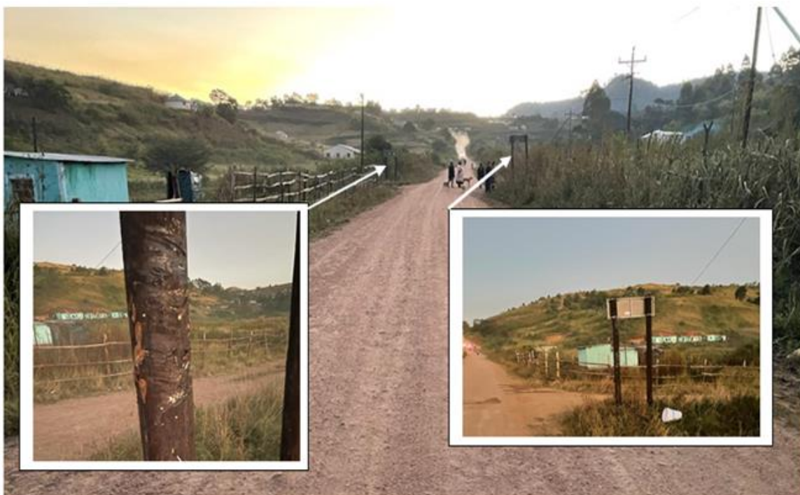
Figure 3: Minor damage to the road sign poles.
