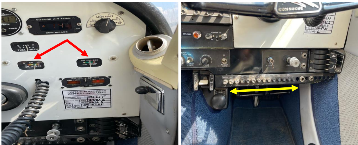
Figures 1/2: The indication of the oil pressure and the oil temperature within limits (green arch), (left picture). A picture of the instruments panel showing all the CBs in pressed-in position (right picture). (Source: AME)
