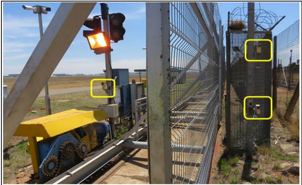
Figure 14: The Echo gate with three of the safety beams visible in the yellow windows.
