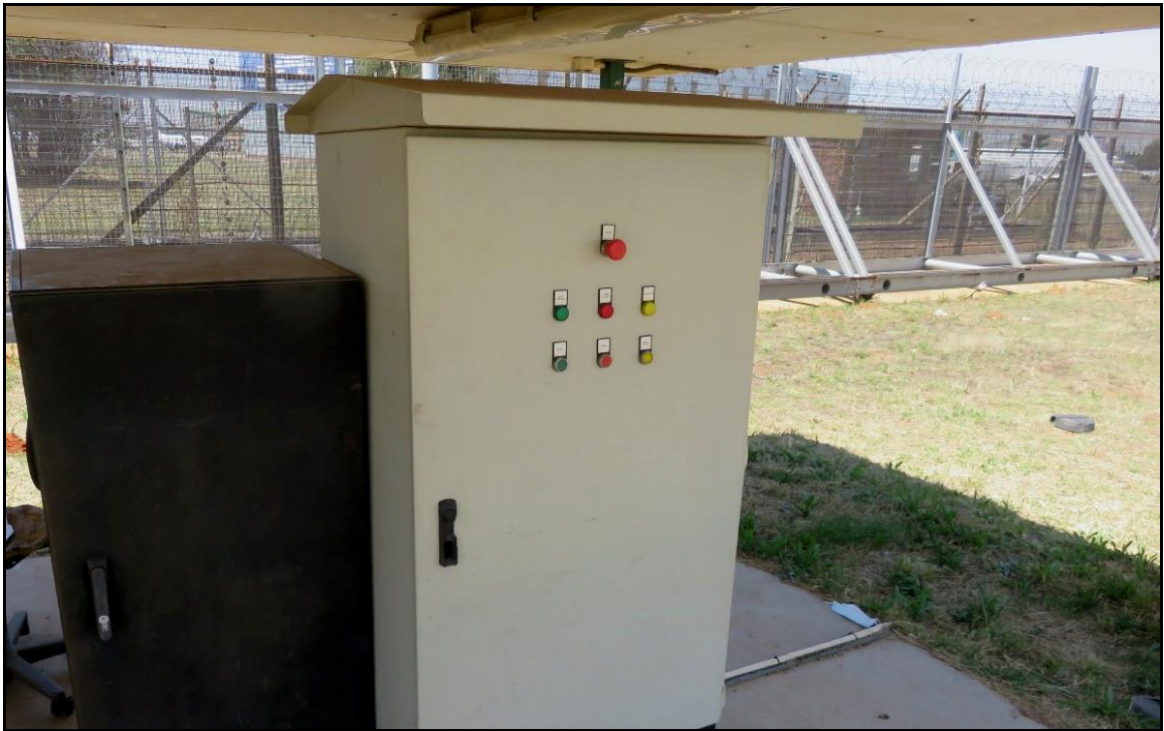
Figure 16: Gate control box installed at the guard house at the Echo gate.
