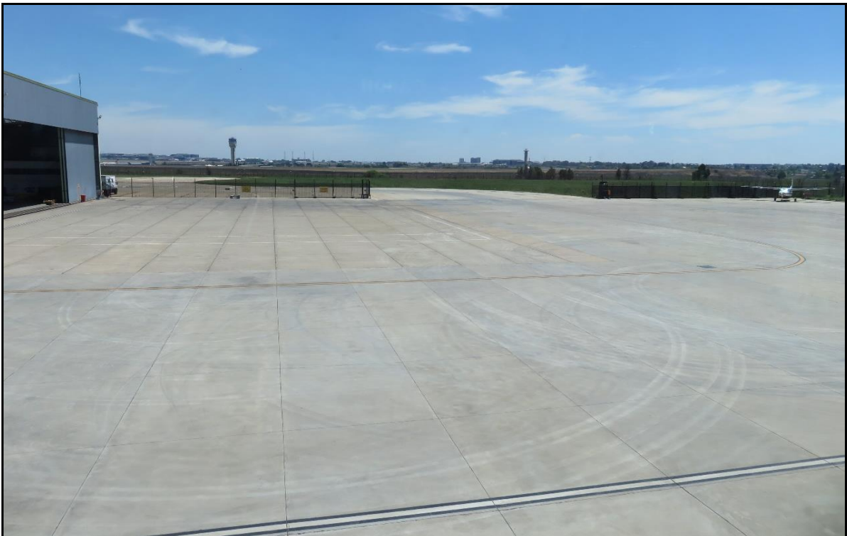
Figure 21: The FBO apron area. The photograph was taken from the FBO centre.
