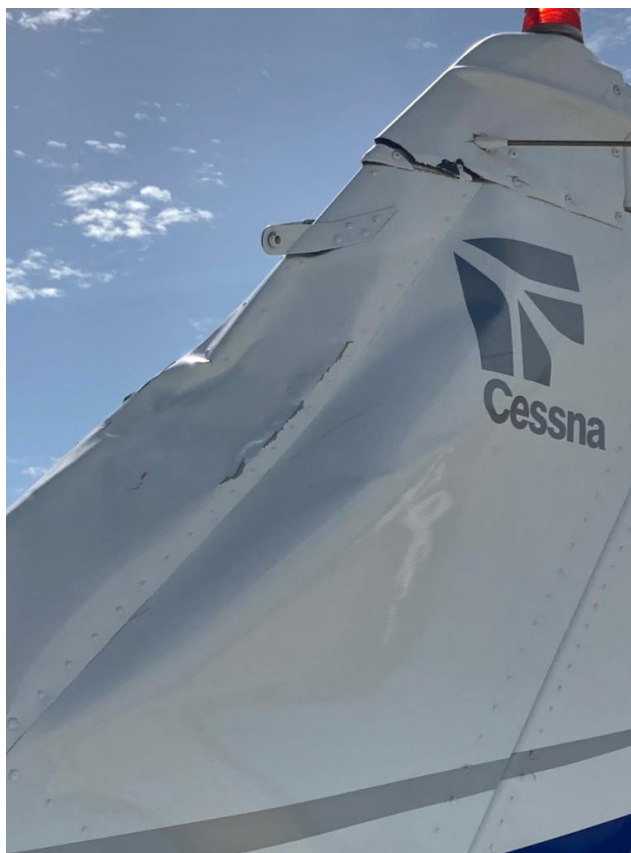
Figure 1: Damaged vertical stabiliser. (Source: Pilot)
