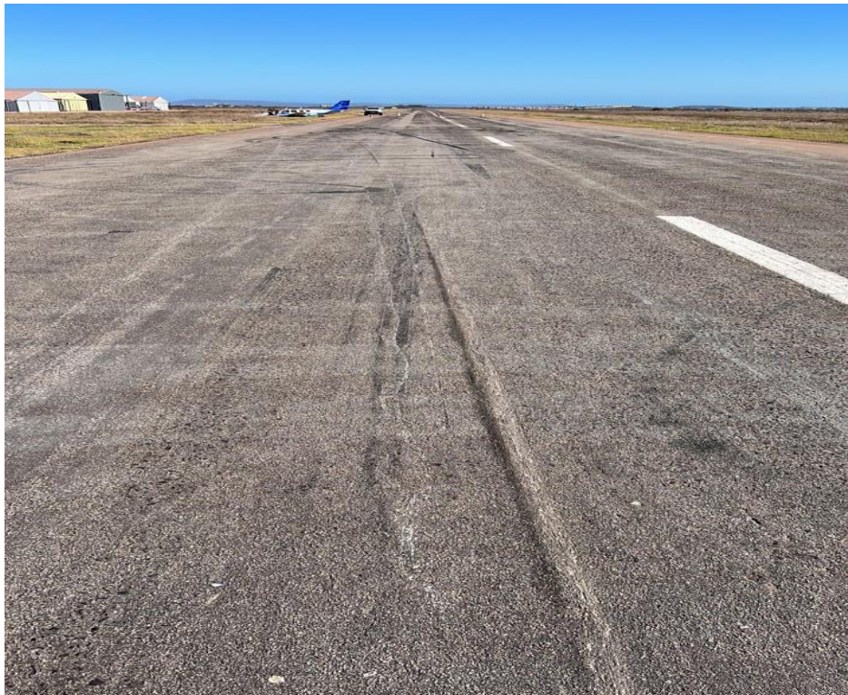
Figure 3: The skid marks on Runway 20. (Source: Owner)
