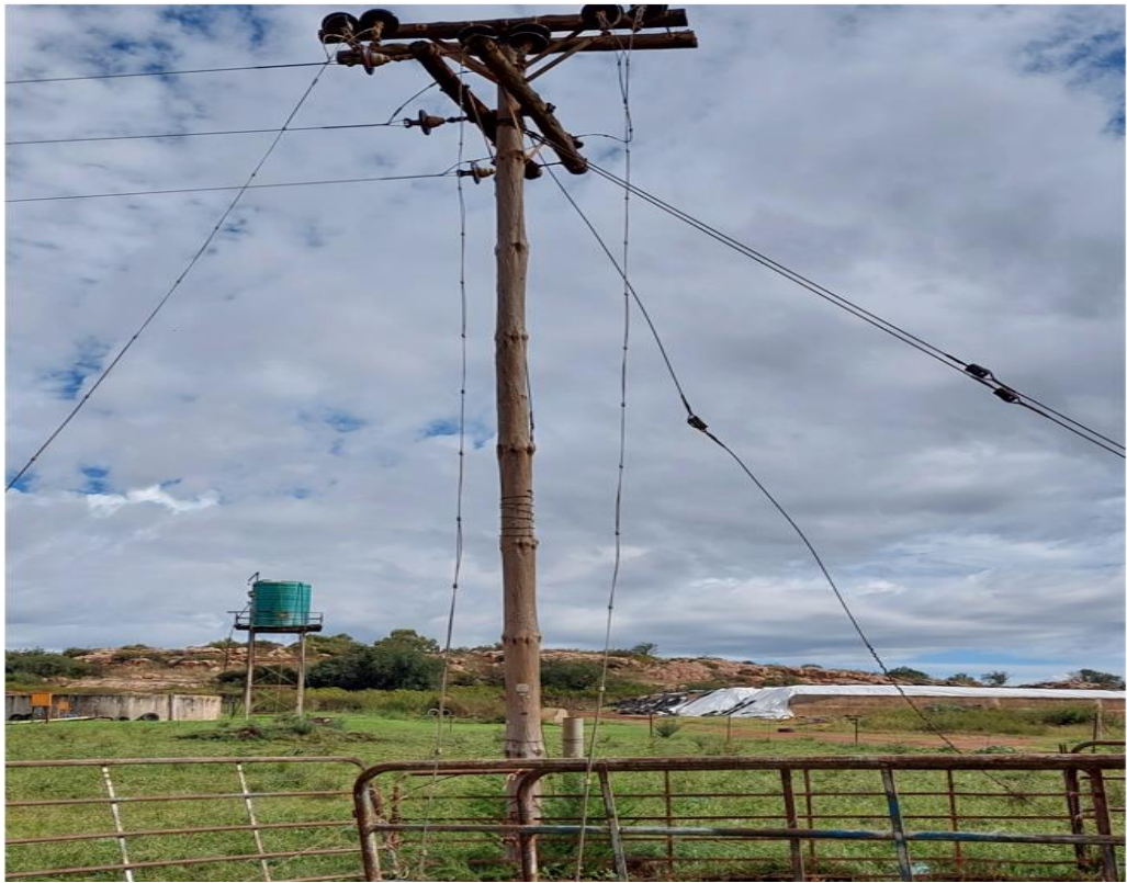
Figure 5: The electric cable pole.
