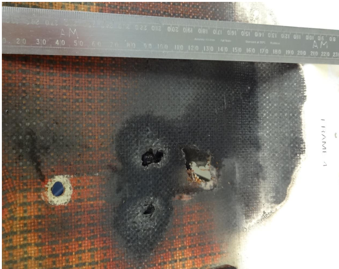
Figure 5: Burn damage sustained to the ceiling panel. (Source: Zenith Aviation)
