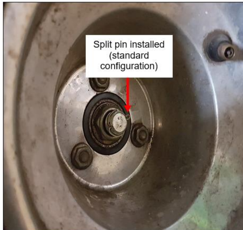
Figure 2: Image of the Bantam B22J wheel secured by a split pin after the serious incident. (Source: Leading-Edge Maintenance)
