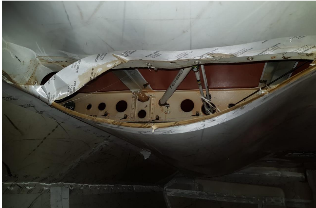
Figure 12: View of the partially collapsed ceiling in the cargo hold.
