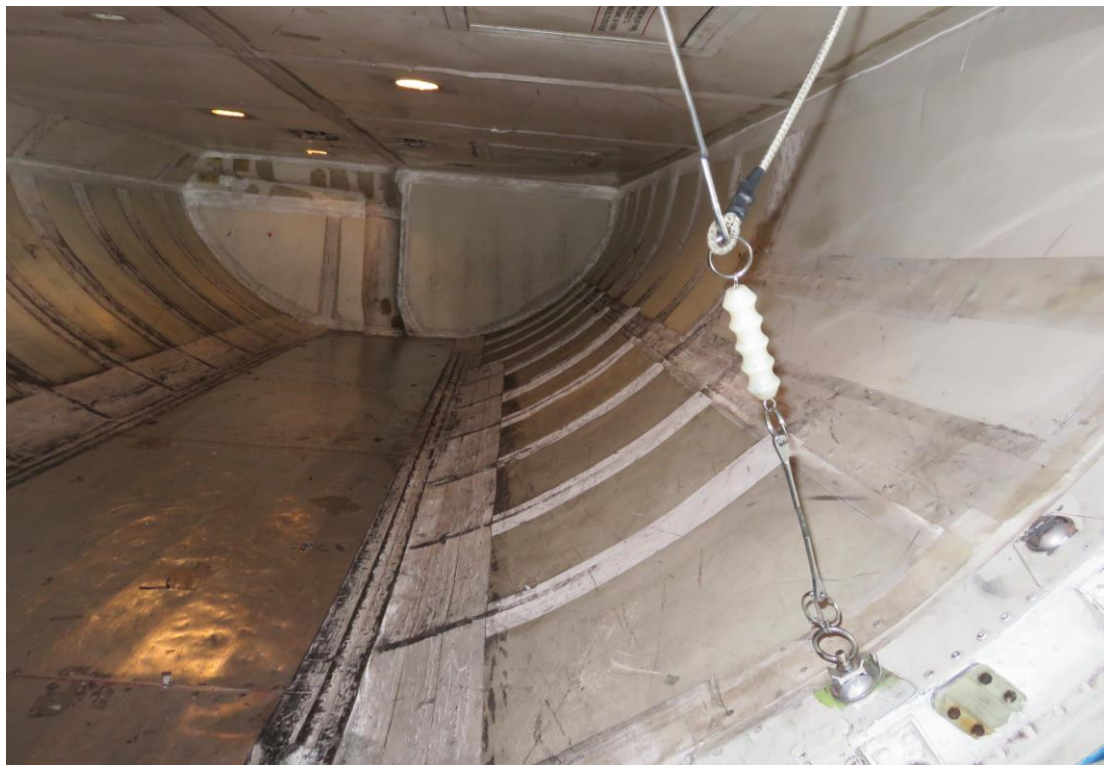
Figure 17: A view of the aft cargo compartment forward section with safety nets removed.
