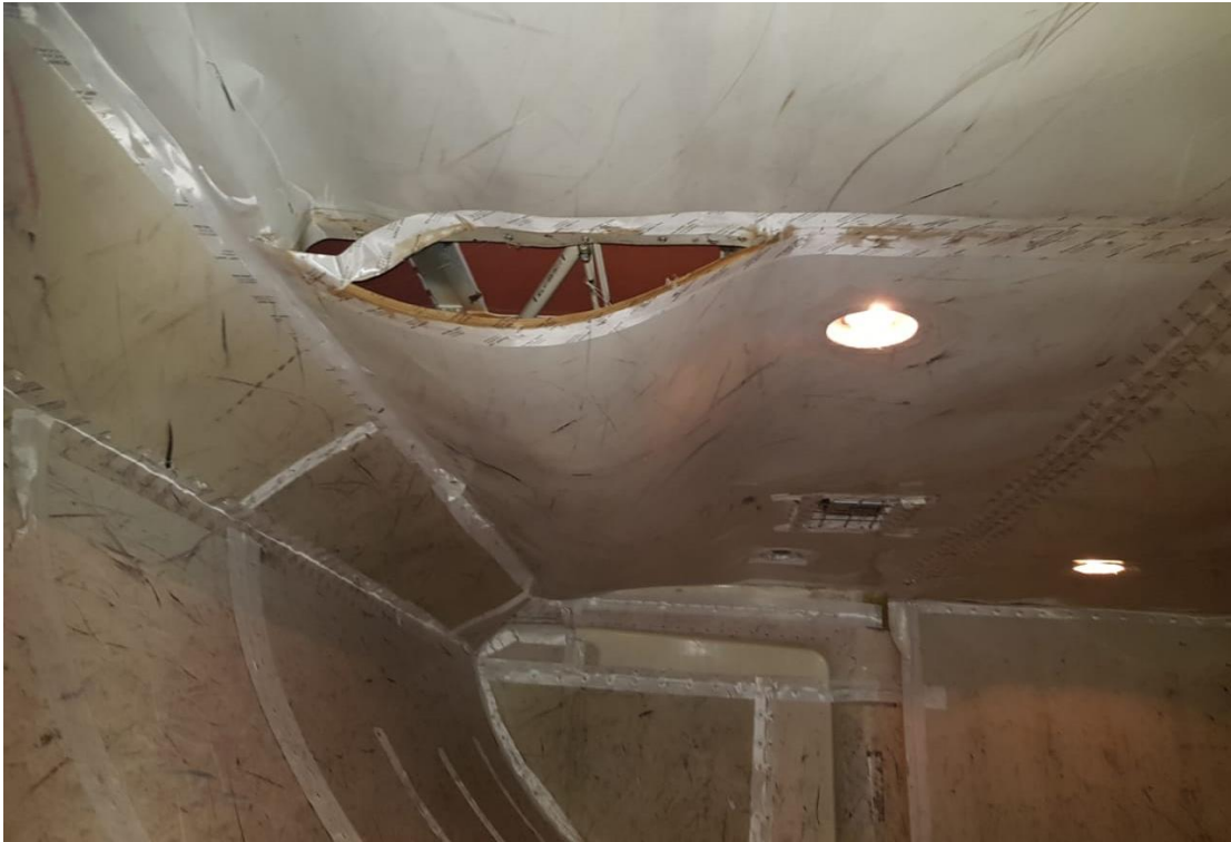
Figure 11: The interior of the aft cargo hold area with a partially collapsed ceiling.
