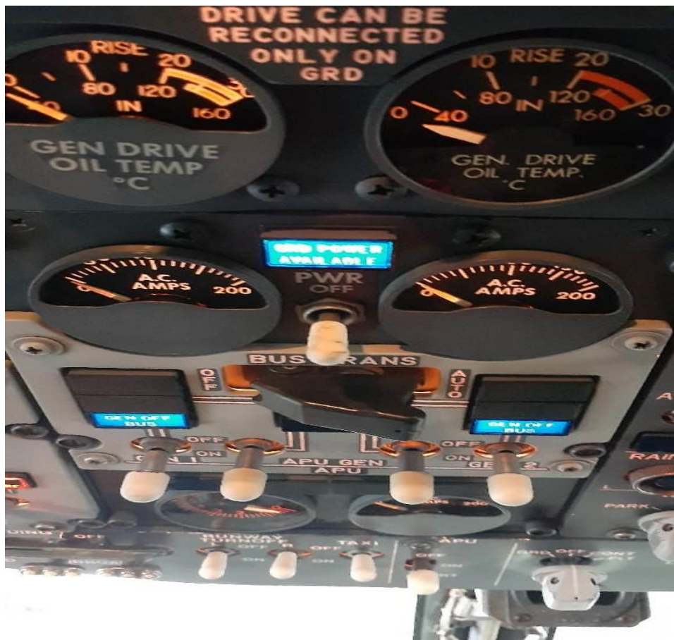
Figure 7: Overhead Electrical Panel
