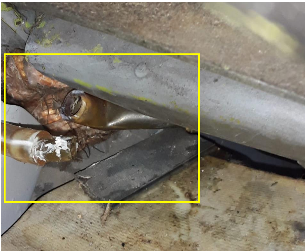
Figure 5: A dislodge water drain tube as found during an inspection by the AMO. (Source: Safair Aviation Safety Division)
