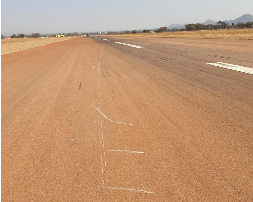
Figure 1: Propeller strike markings on Runway 29 at FAWB.
