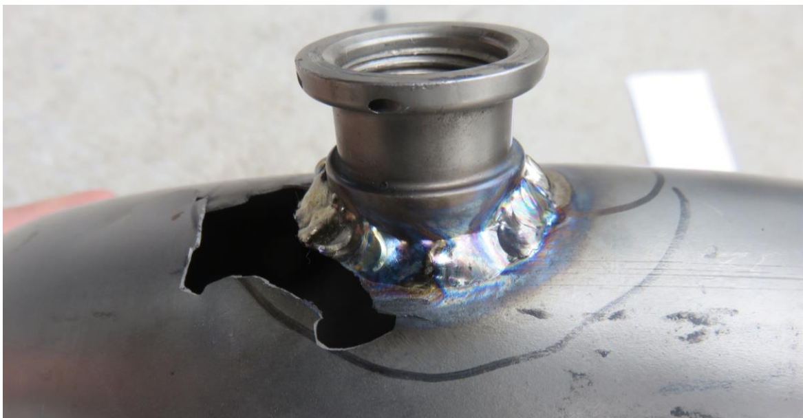
Figure 9: Closer view of the discoloured welding around the circumference of the nipple.
