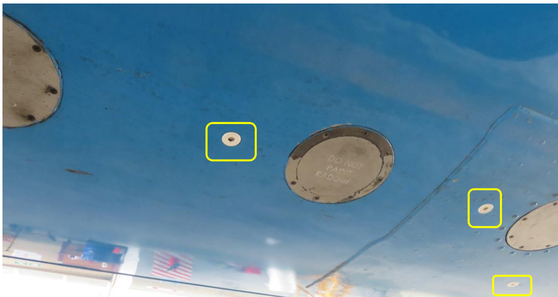
Figure 20: The bilge valves mounted at various places on the lower fuselage.
