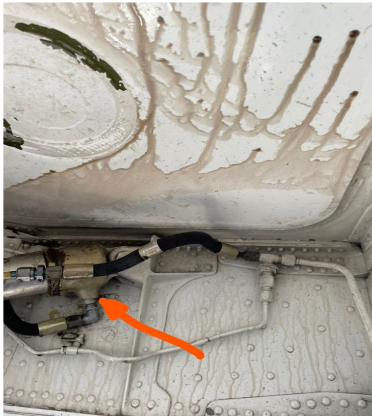
Figure 2: Position of the hydraulic fluid seal in the left main gear wheel well. (Source: Operator)
