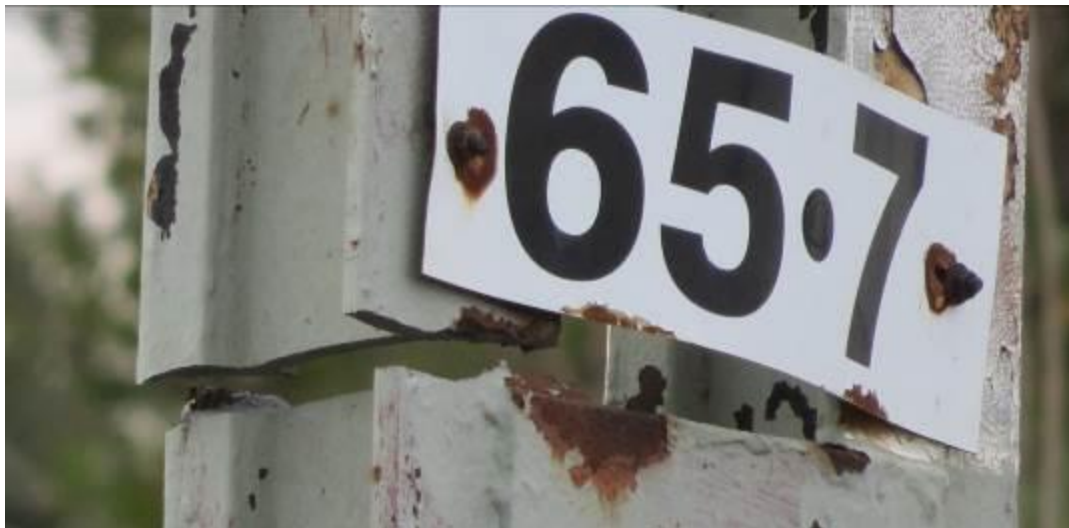
Figure 2: A close-up view of the pylon that fractured
