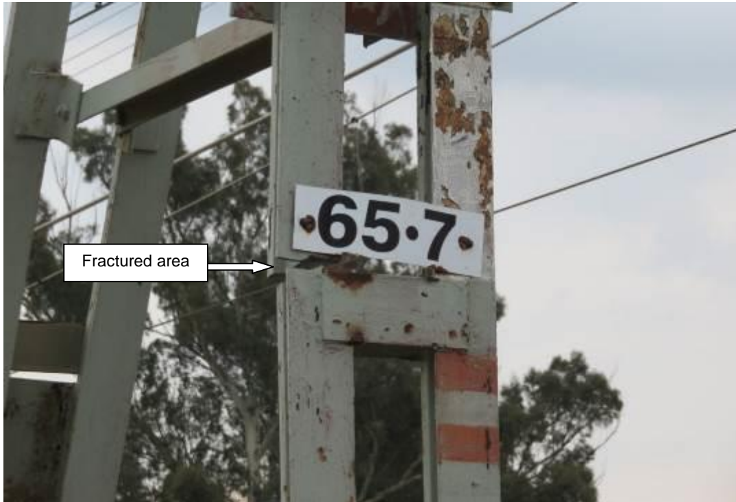
Figure 1: The railroad electrical support pylon that fractured and needed to be replaced
