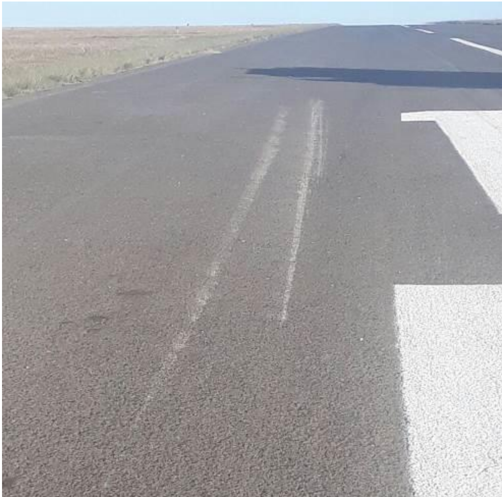
Figure 9: Scrape markings from the left wing at the threshold of Runway 17
