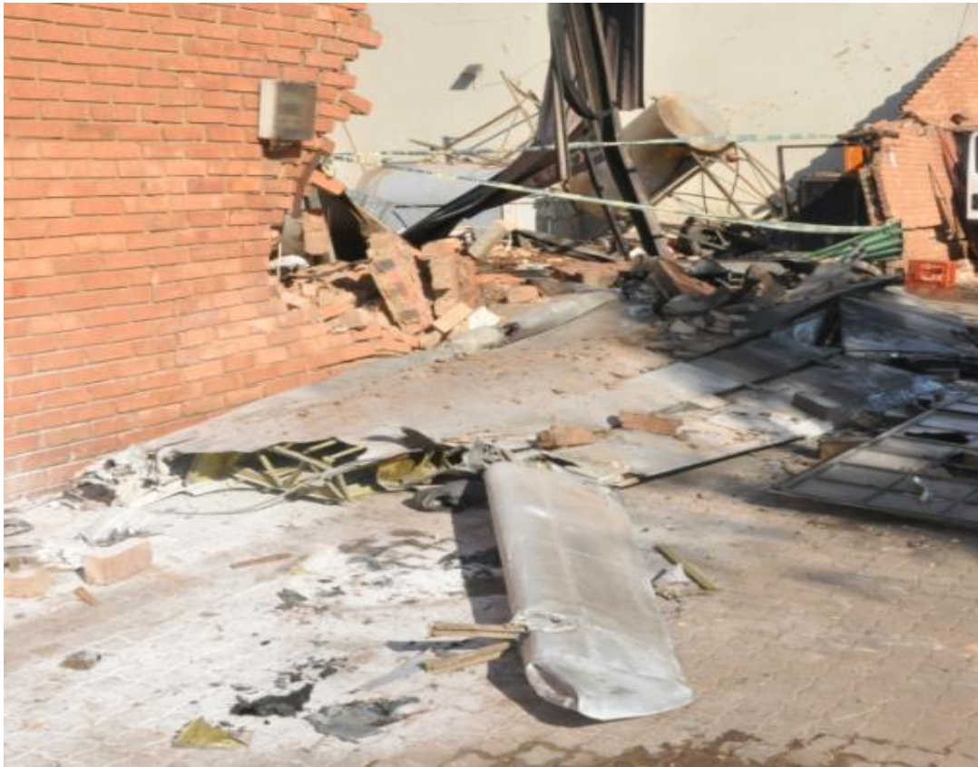
Figure 20: The left wing out-board section and part of the building damaged by the aircraft during the accident sequence.
