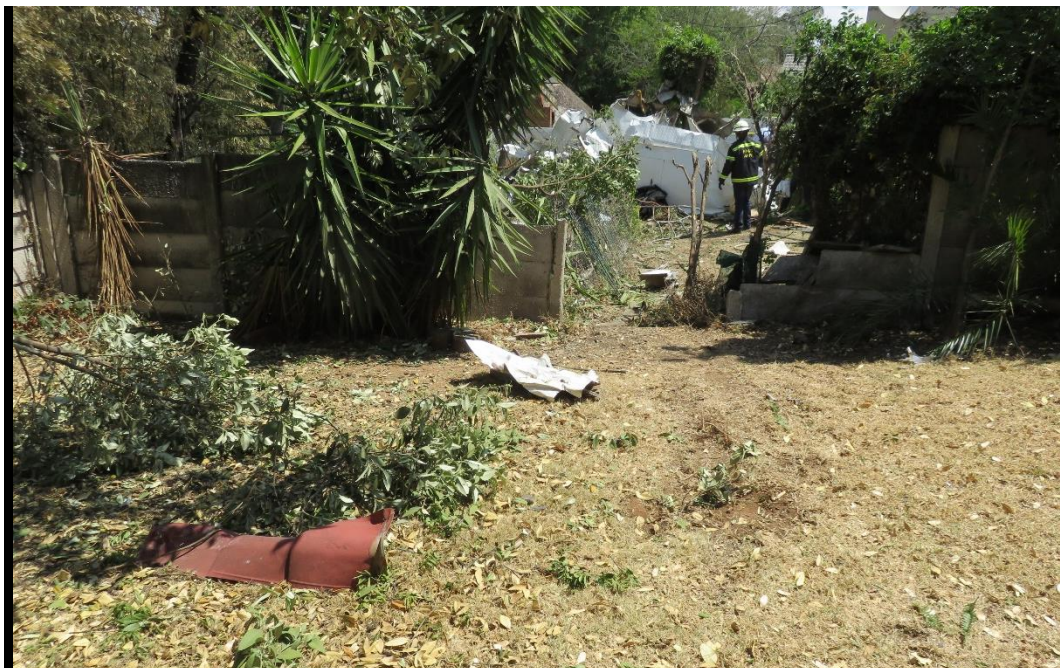
Figure 10: Damage to the precast wall and a piece from the damaged roof
