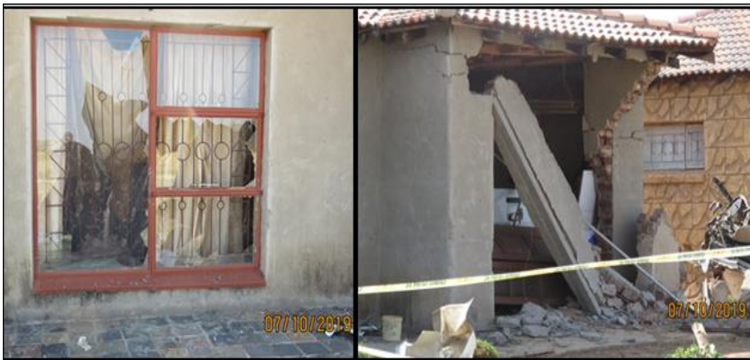
Figures 3 and 4: Damage caused to the window of the house, the garage door and the parameter wall.
