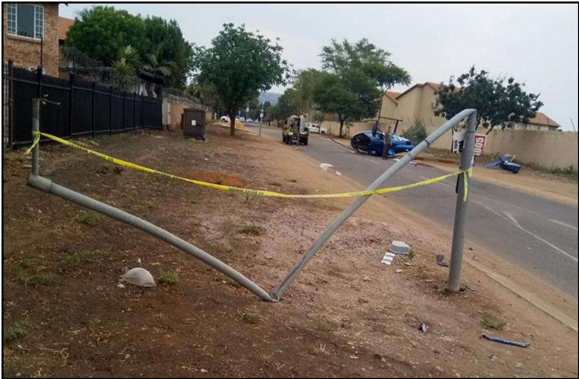
Figure 3: The damaged streetlight pole.
