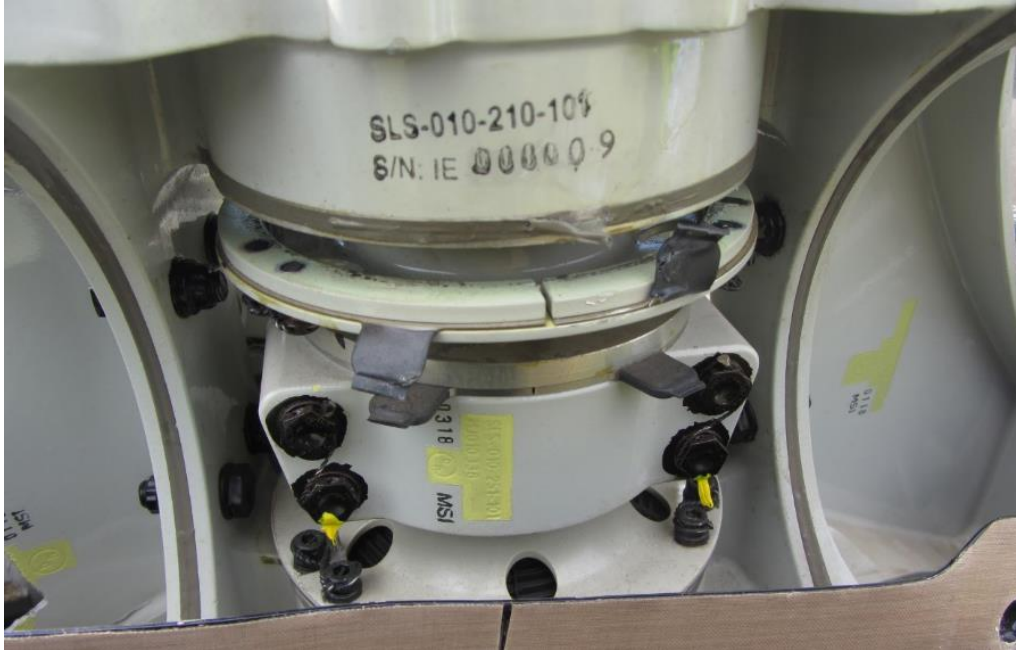
Figure 13: Damaged transmission mounting.
