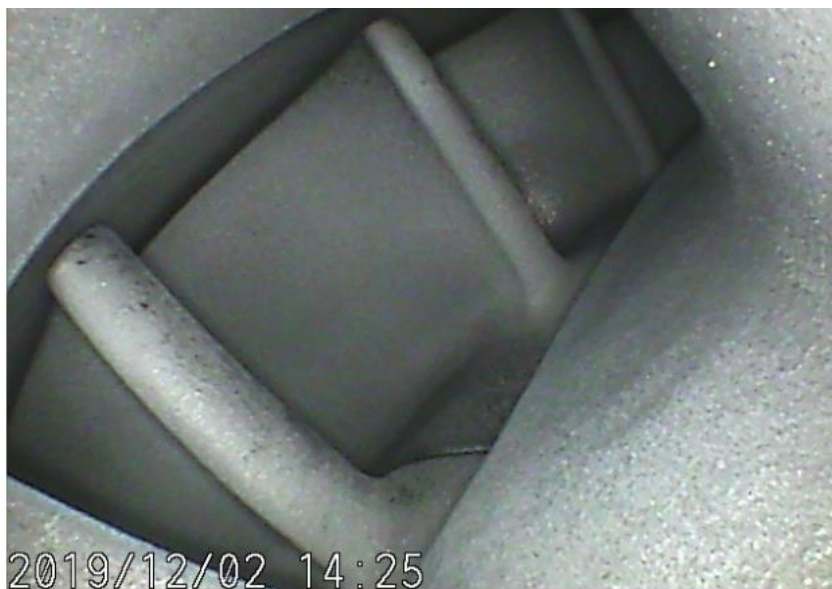
Figure 21: The gas generator turbine.
