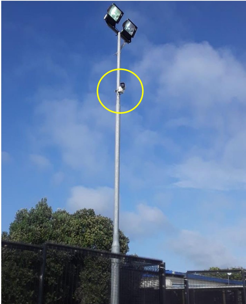
Figure 13: The flood light next to the apron at FAPG with the CCTV camera attached.
