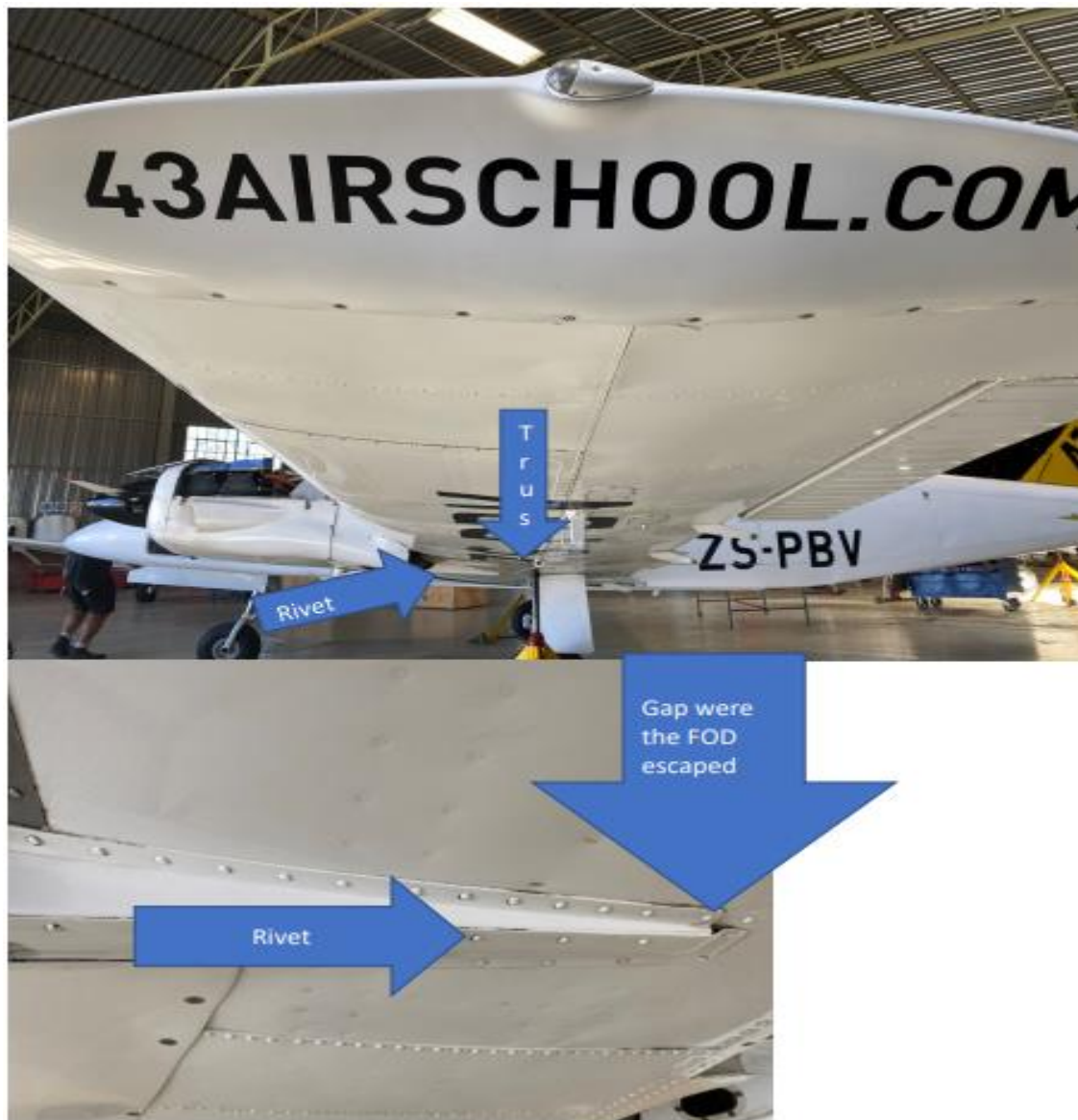
Figures 1 (top) and 2 (bottom): The left underwing showing the place where the rivet detached/loosen.
