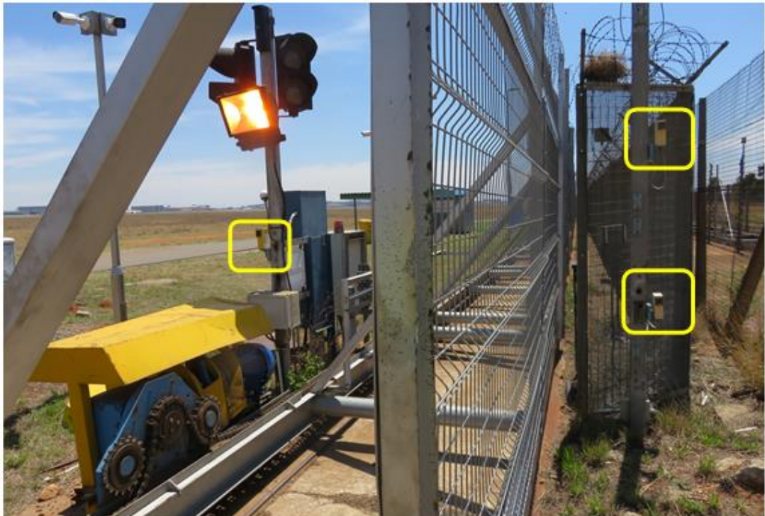
Figure 12: The Echo gate with three of the safety beams visible in the yellow windows.
