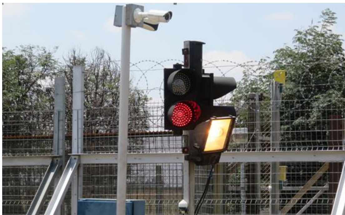
Figure 16: The traffic light at the gate open position.
