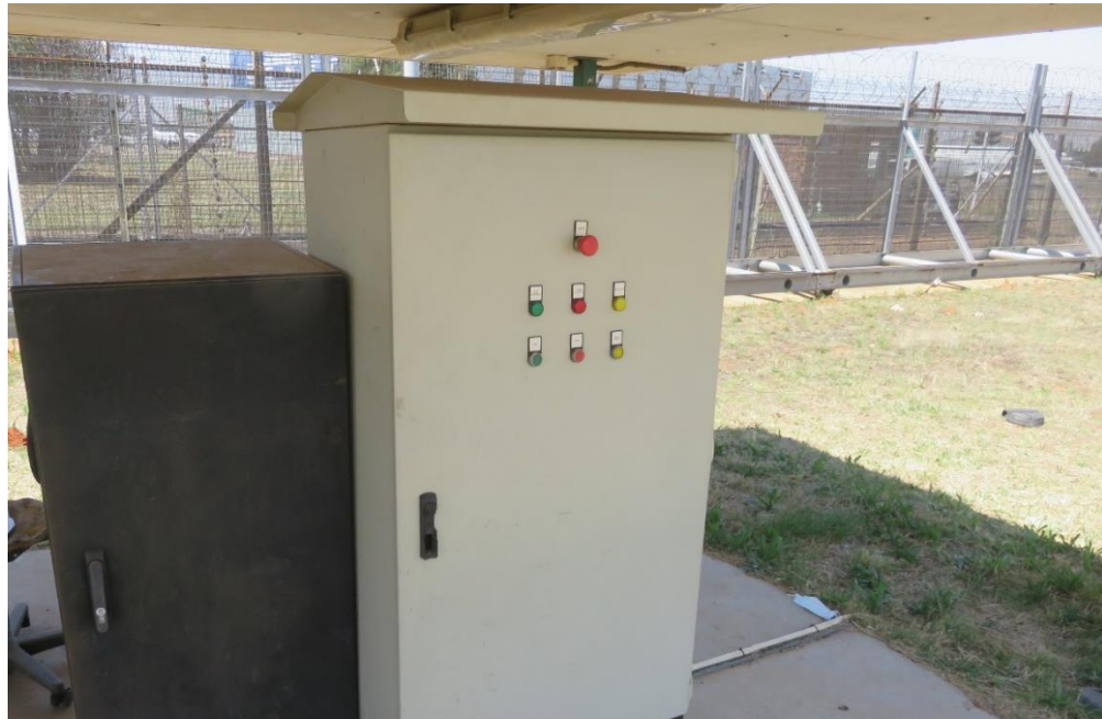
Figure 14: The gate control box installed at the guard house at Echo gate.
