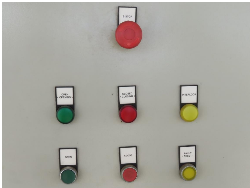
Figure 15: The gate control box with the E-STOP button at the top.
