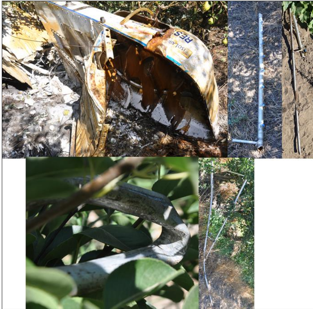
Figure 15: Damaged and scattered IsoLair spray system components.
