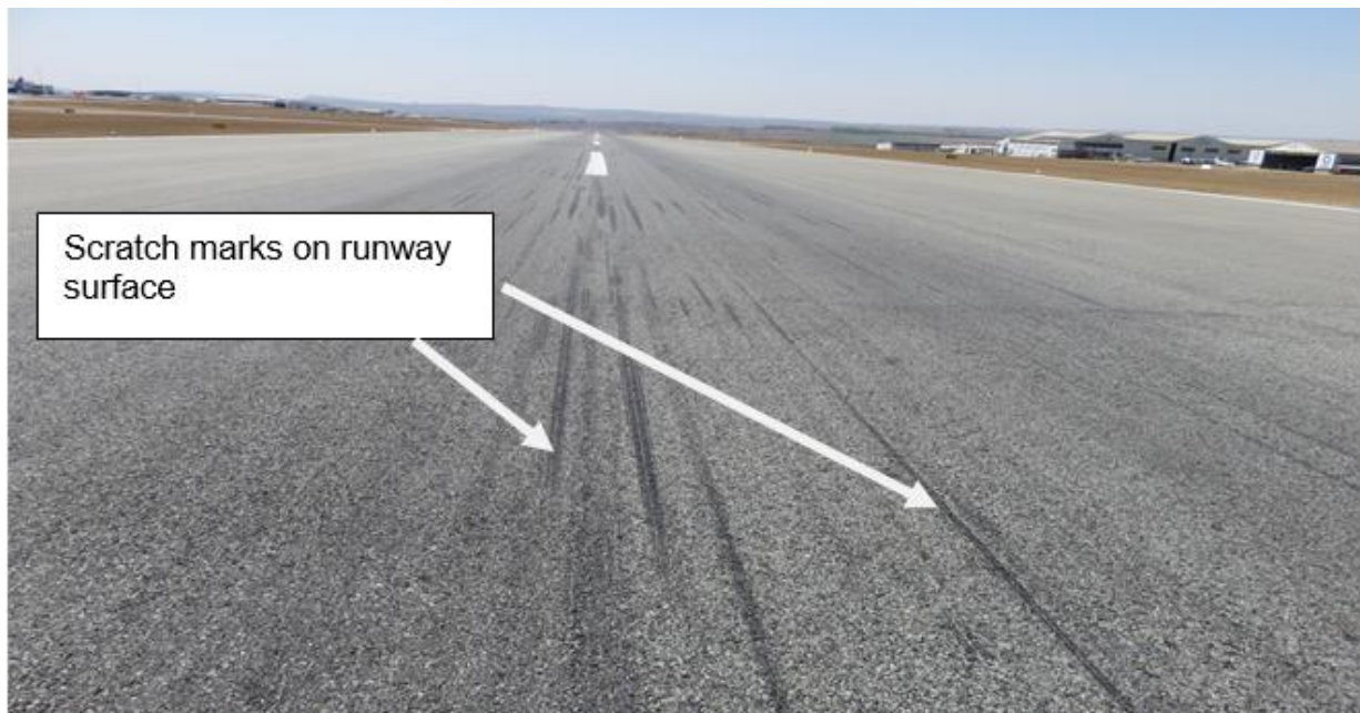
Figure 5: Scratch marks on runway surface at FALA.
