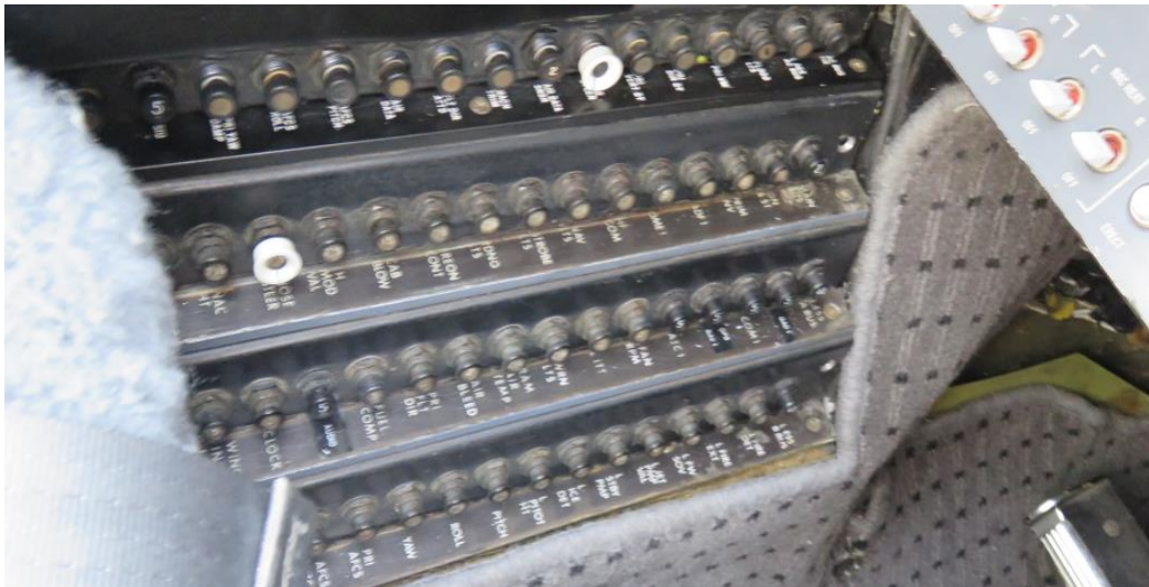
Figure 11: All circuit breakers were in a closed position.
