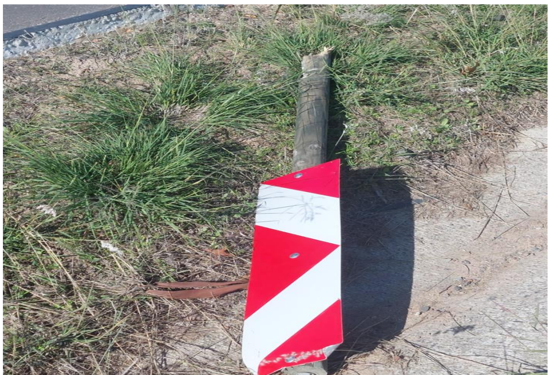
Figure 4: The severed road sign pole.
